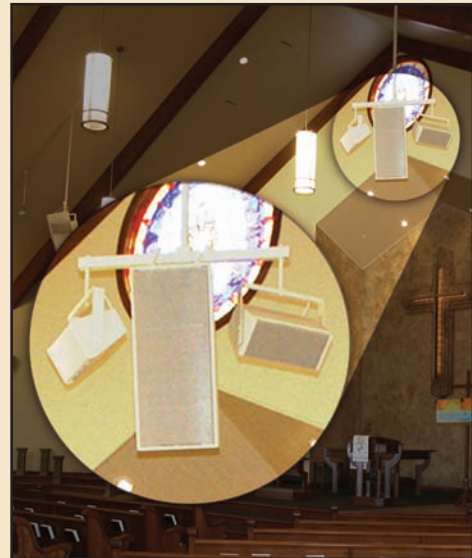
Figure 4 Overhead loudspeaker mounting is a safety hot spot.
